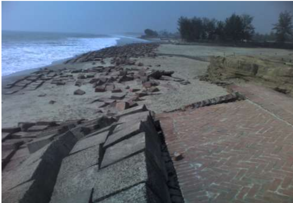
Picture: Save the Sea beach, Cox's Bazaar, the Wonder of the World Hill cutting and Shrimp Hatcheries eroding the beach
